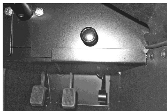
Figure 110: Heater control location
